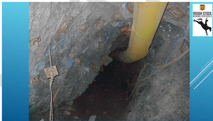
Vent Bag in a Production Heading (area)
